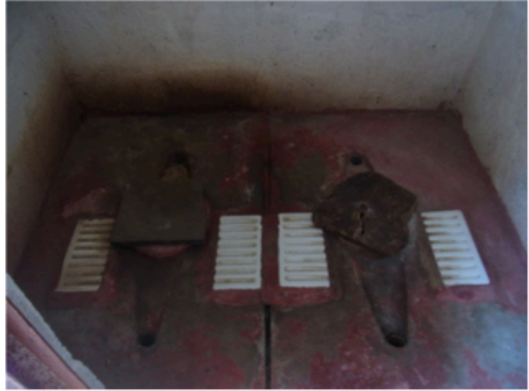
Unclean EcoSan toilets using tiles as covers in Amadaikuppam
