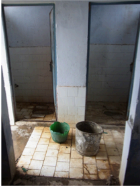
Dysfunctional toilets in Soolegunda school, Krishnagiri
