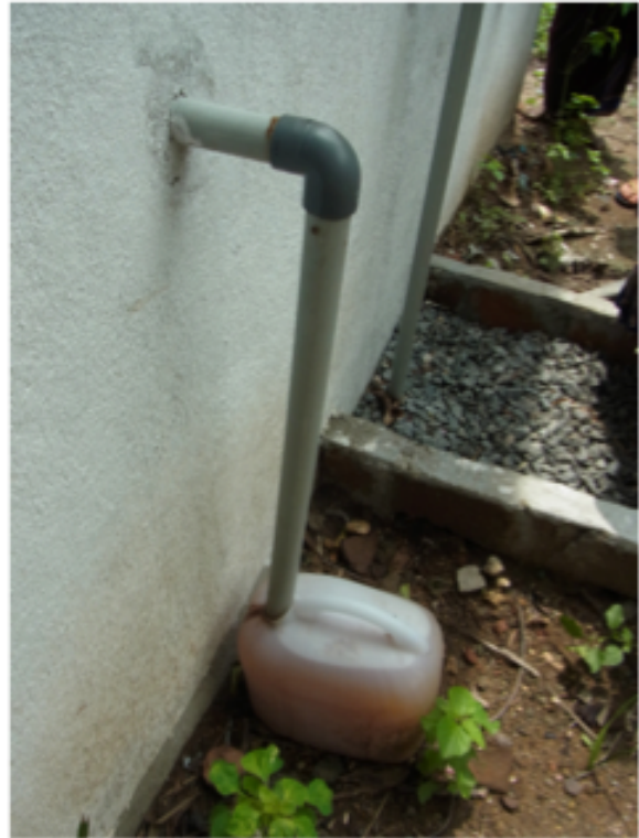
Urine diversion for crop application and anal cleansing water filtration system into reed bed.
